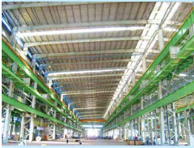
Multi-Level Crane Beam
