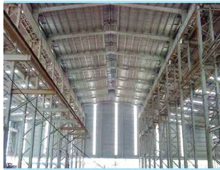
AHT Steel Mill - 1,000 MT
