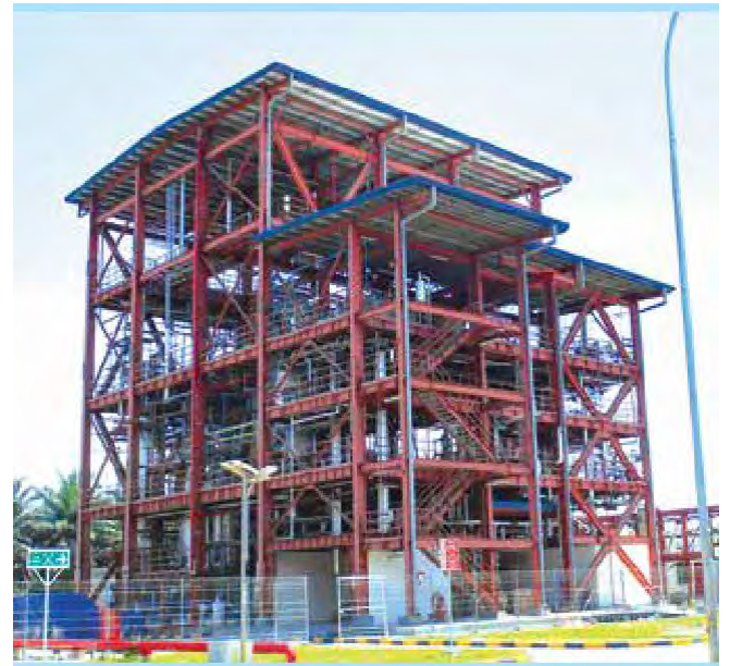
Hydrogenation Plant (Indonesia)
