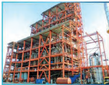
Fatty Acid Plant
